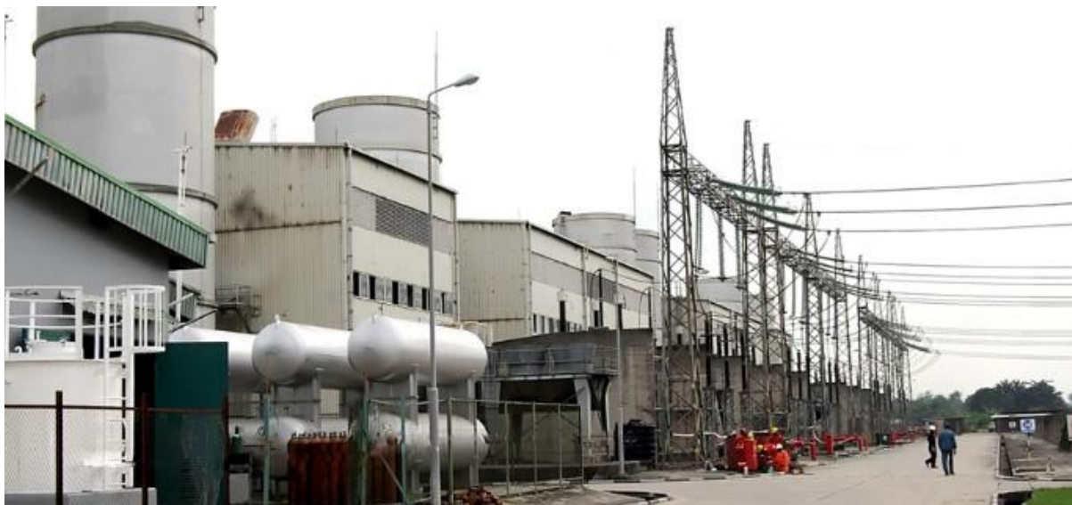
Figure 2.1: A Picture of Ughelli Electric Power Station; One of the above Six Electricity Generation Companies in Nigeria
